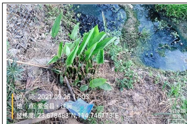
图3.5-3 污水主管破损
